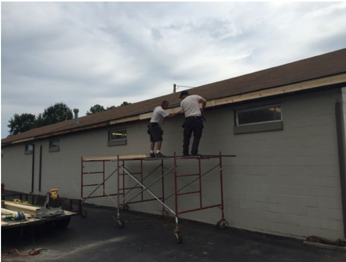
Work being done to replace the rotten roof on the holding house.
